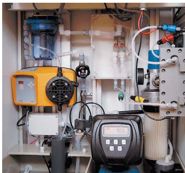
Figure 2: View of the interior of the generator
